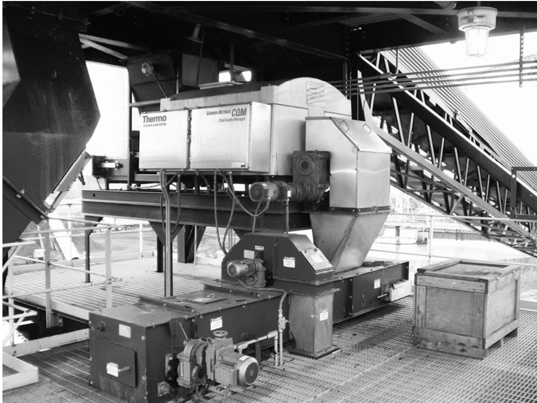
Figure 4. Typical Sample Stream On-line PGNAA Coal Analyzer Installation
