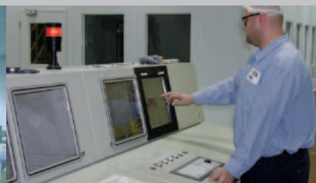
The Operator Control Panel
